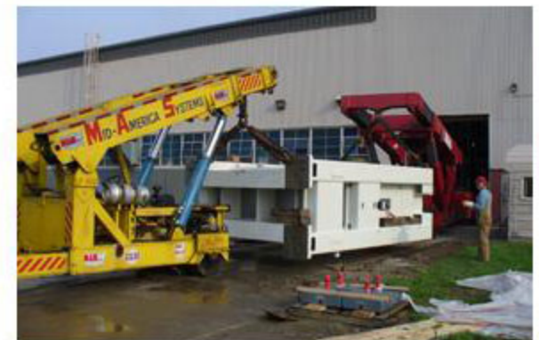
Two twinlifts at work installing a press in low head room facility
