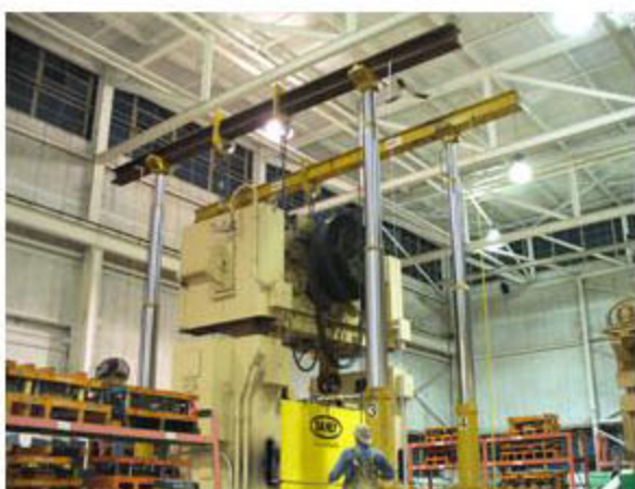
Press installation with gantry
